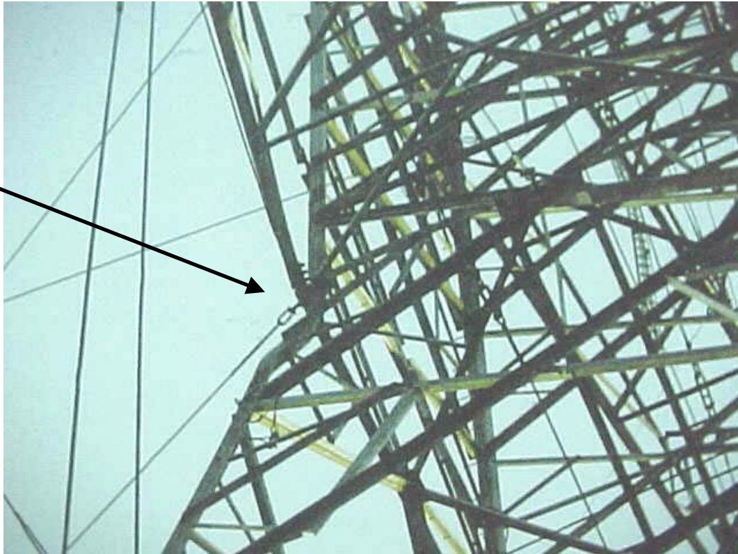
Figure 12 – Failure at 90 % loading
