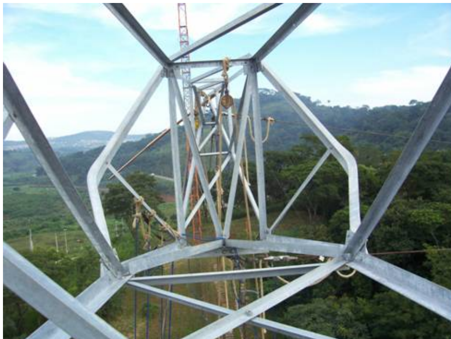
Figure 15 – Failure at 100 % loading
