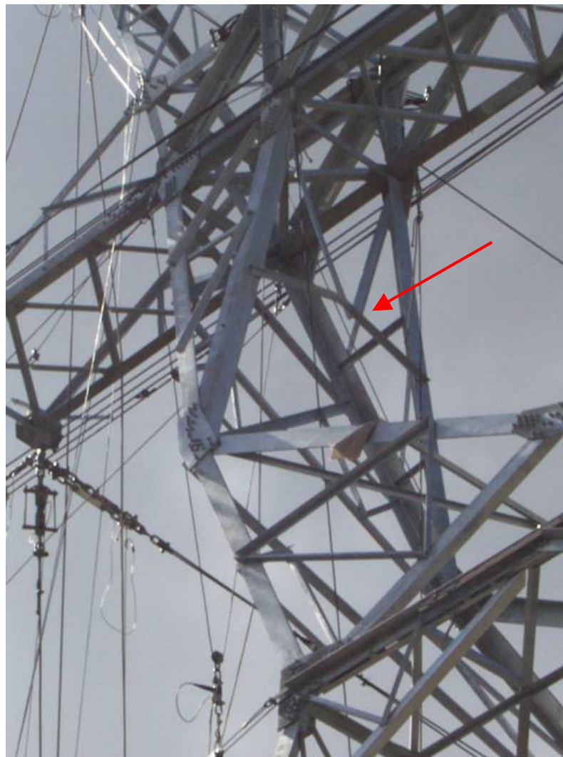
Figure 16 – Failure of redundant member
