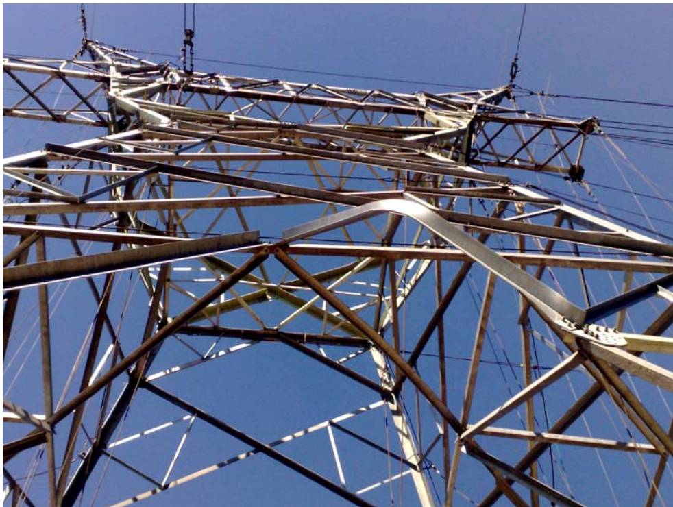
Figure 7 – Member fail by compression
