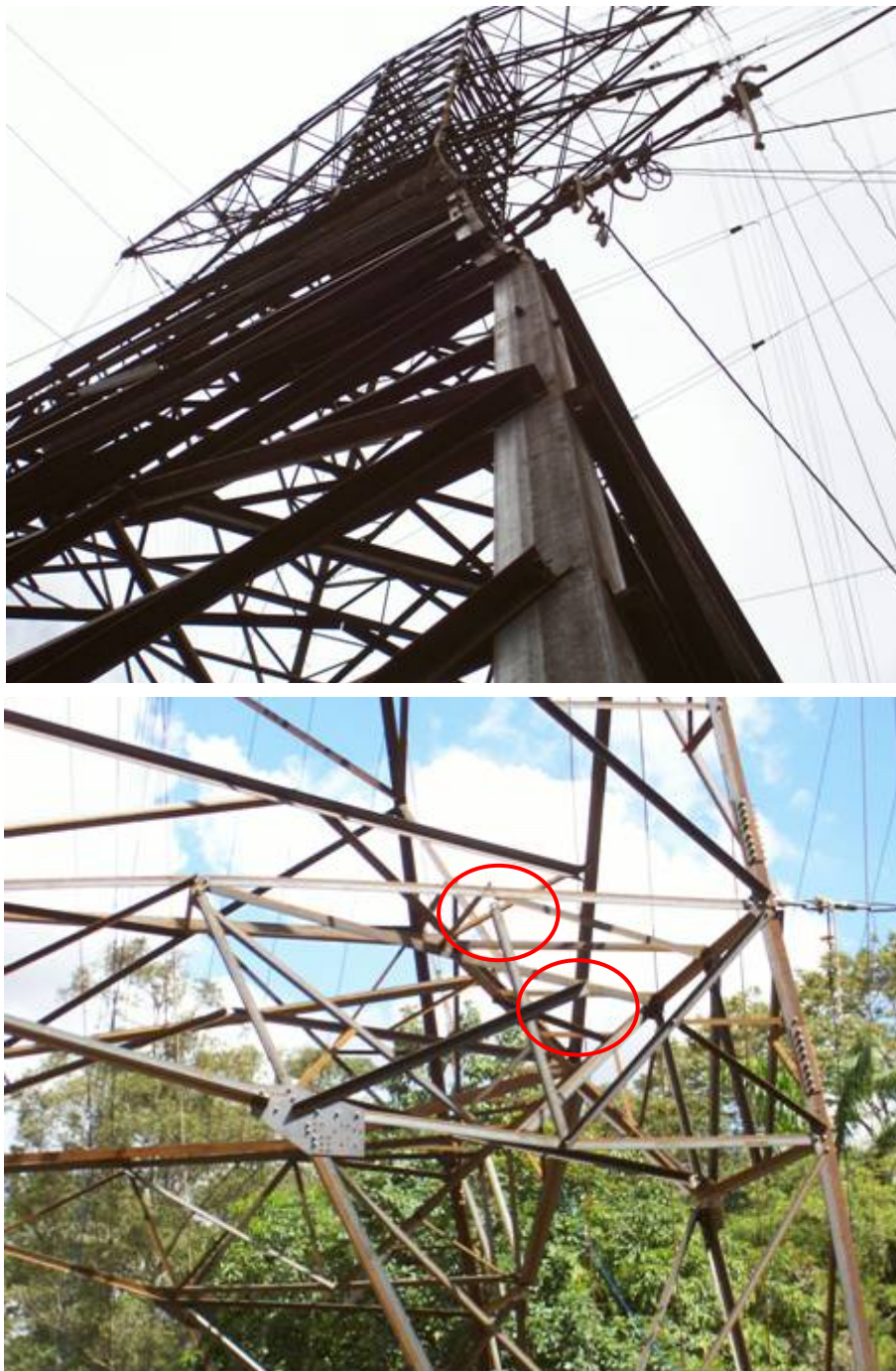
Figure 10 – Failure at 75 % loading
