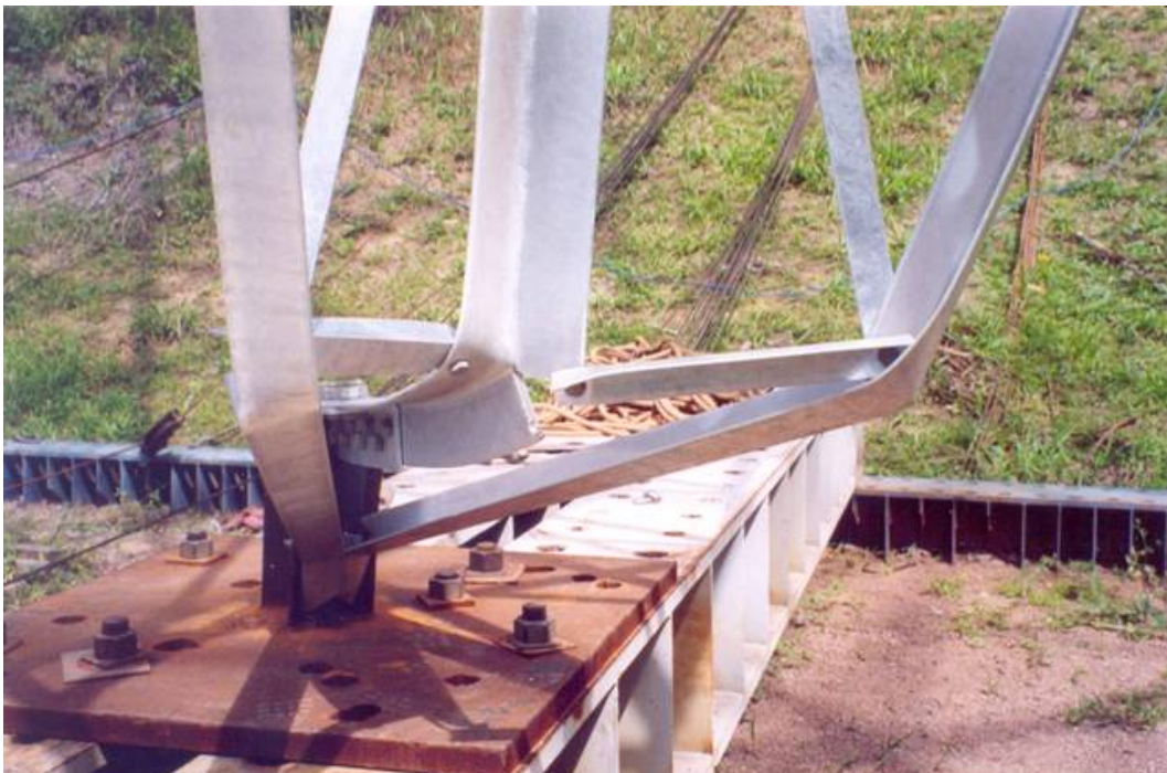
Figure 5 – Buckling on tower leg extension
