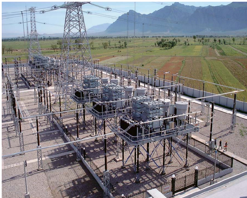
Figure 2.17: Dafang (China): 500kV, 2x372Mvar series compensation (source ABB)
