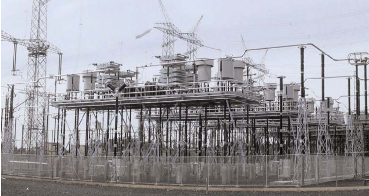
Figure 2.14: Furnas (Brazil) 765kV, 1056Mvar series capacitors (source ABB)
