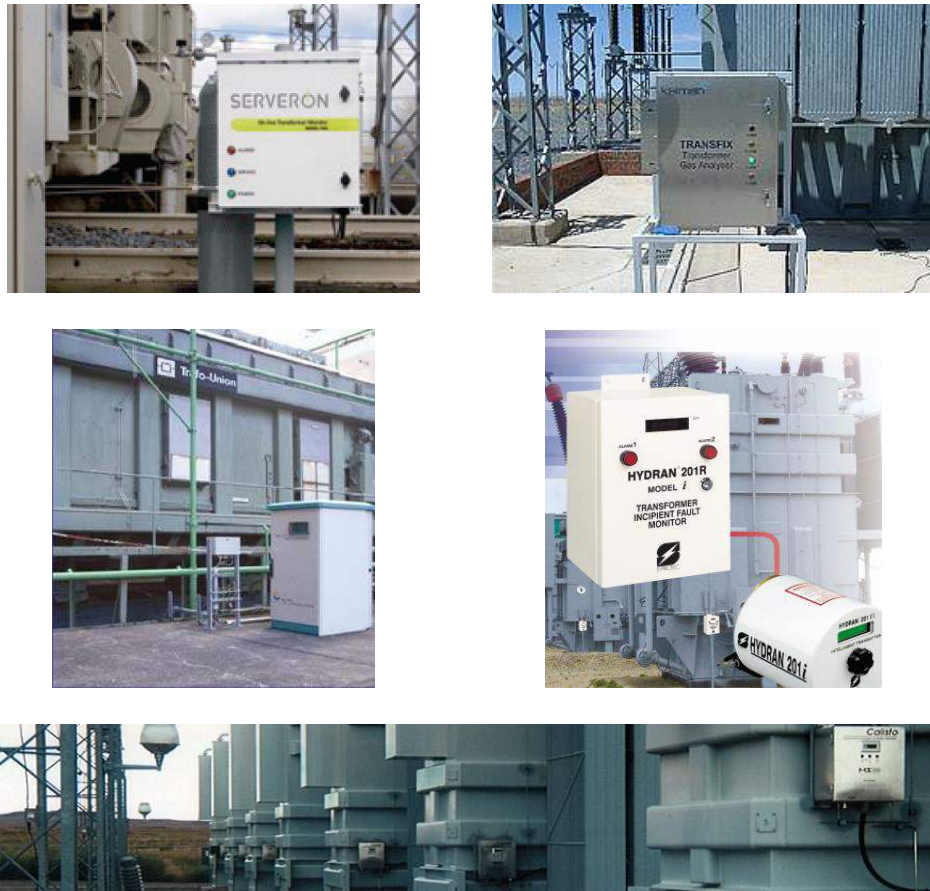
Figure 1: Examples of installation of on-line monitors
