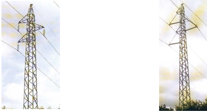
Figure 11: Uprating a 66 kV lines to 220 kV with minimal cost and construction time
