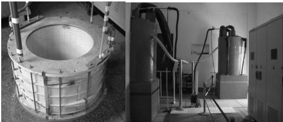
Fig. 5.5: Left – HTS coil for diode bridge type SCFCL Right – Installation of 10.5 kV, 1.5 kA diode bridge type SCFCL at substation in Hunan, China
