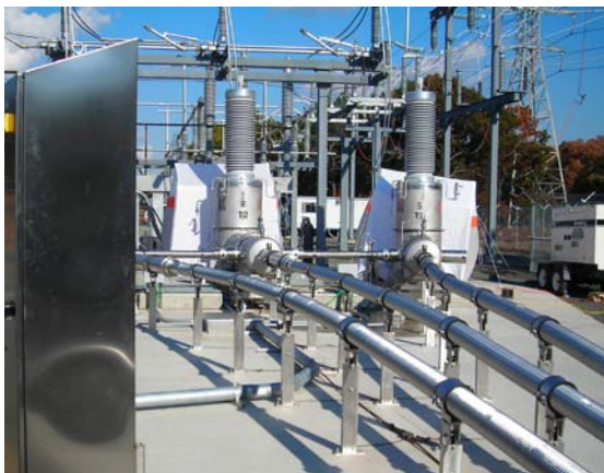
Fig. 4.5: 138 kV HTS cable with terminations
