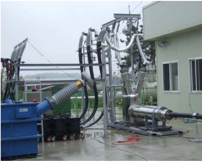
Fig. 4.10: 22.9 kV HTS cable with termination (3 phase in 1 termination)
