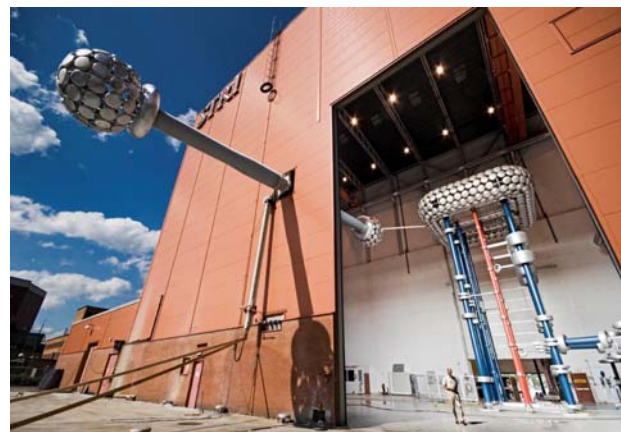
Figure 3.6- 800 kV DC wall bushing during tests at STRI, Ludvika (Courtesy ABB)
