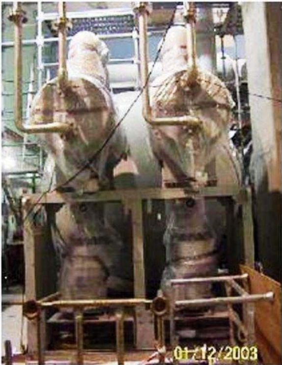
Figure 18: Typical on-site leakage measurement on 330 kV-400 MVA GIT (Water-SF 6 heat exchanger parts)
