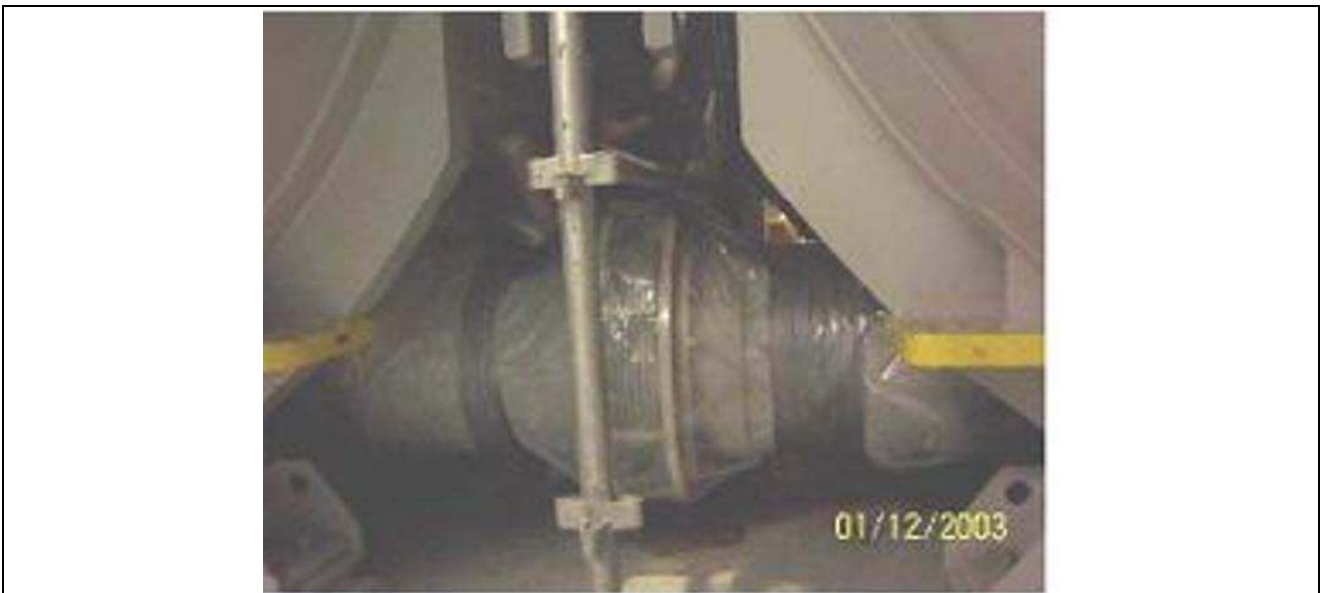
Figure 17: Typical on-site leakage measurement on GIT connection part
