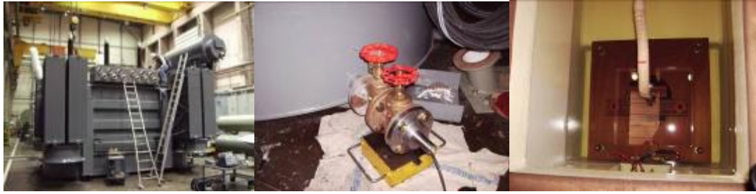
Fig. 5.14: Laboratory setup (left picture) used to simulate the on-site step of the sensitivity check using an internal sensor through the oil valve (middle picture) and injection using a sensor through an opening in the top cover of the transformer (right picture).
