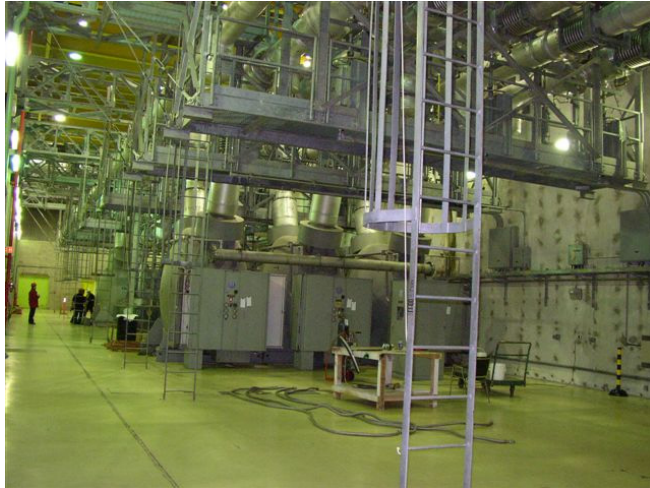
MICA GS Switchyard – Old Breakers
