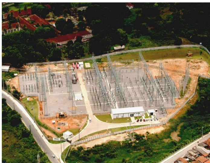
Figure 3 – Aerial view of the Joairam Substation - CHESF
