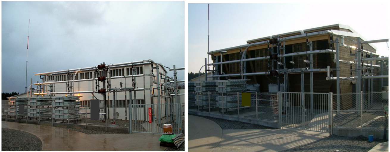
The Static Var Compensator in Poteau Rouge before (left) and after (right) reconstruction
