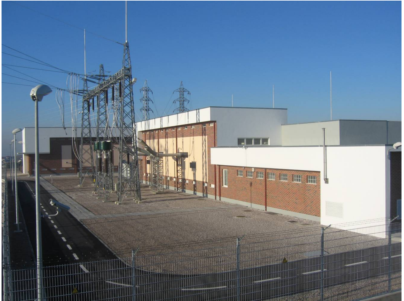
150/60 kV GIS Trafaria Substation. Buildings.
