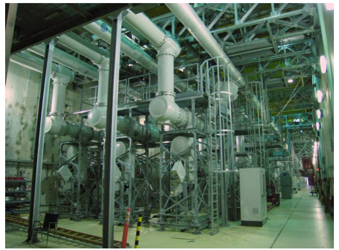
MICA GS New Switchyard
