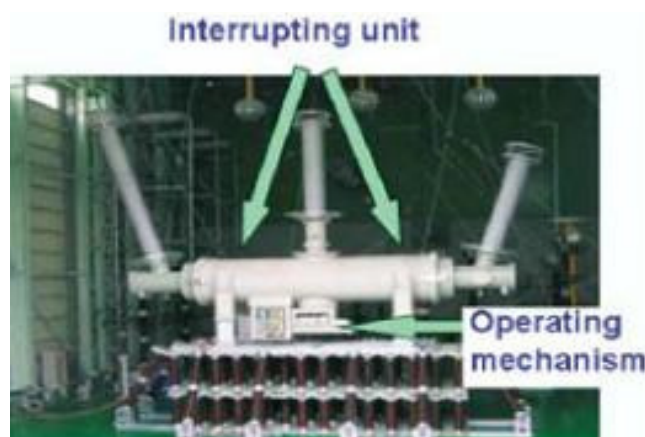
Figure 7.2.9 800 kV full-pole testing in Korea
