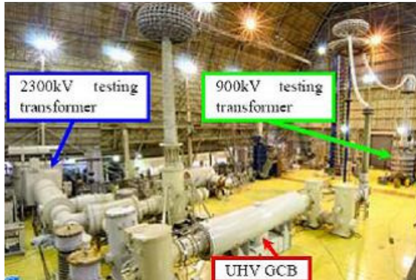
Figure 7.7.4 Set up for UHV dielectric tests in Japan [47]
