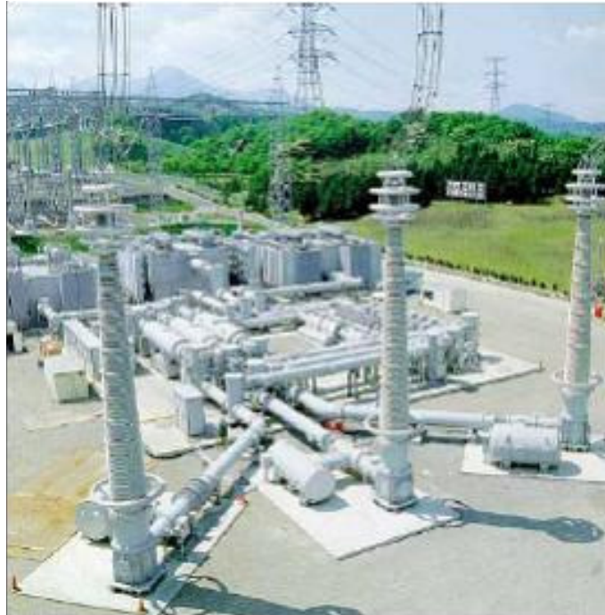
Figure 7.1.3: Japanese Shin-Haruna UHV test station
