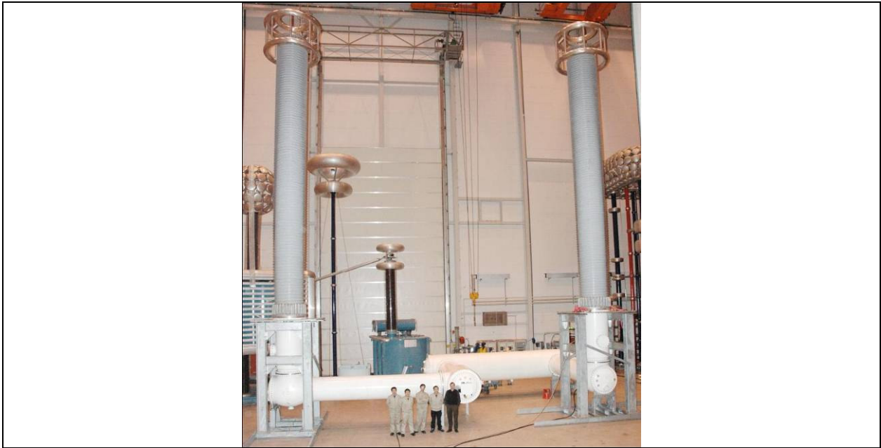
Figure 11-7: GIS module equipped with composite bushings [11.16].
