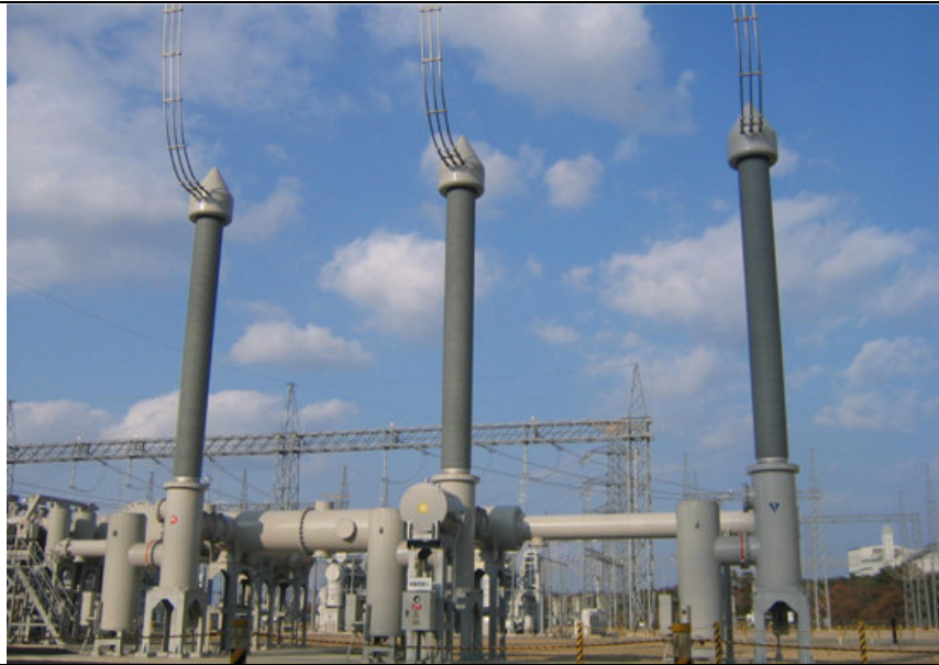
Figure 2-9: 550 kV Gas Insulated Substation
