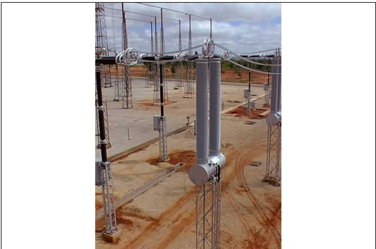
Figure 11-8: 800 kV current transformer installed in Brazil
