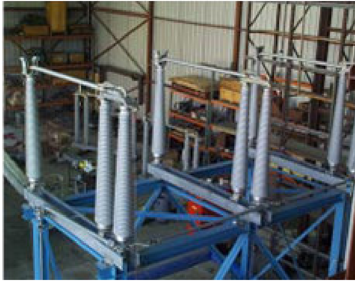
Figure A7-1.1: 242 kV disconnect switch mounted on conical composite insulators during the shake table test. The assembly also included the three phase pedestal
