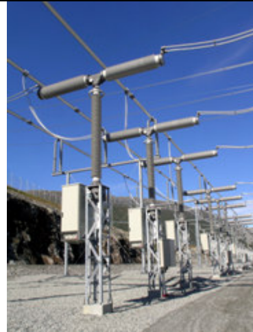
b) Composites on live tank circuit-breaker
