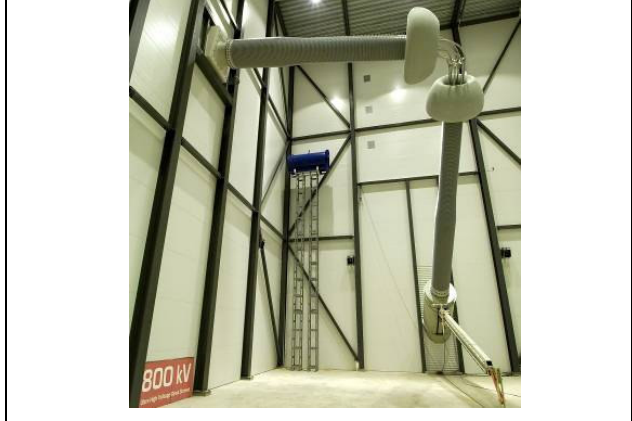
c) Wall and transformer bushing
