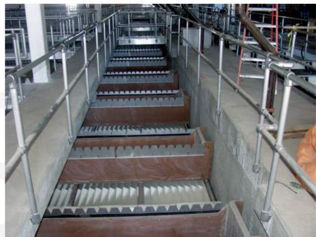
Fig. 6.11a—UHPC troughs for the Gold Bar Wastewater Treatment Plant, Edmonton, AB, Canada (McCraven 2007).
