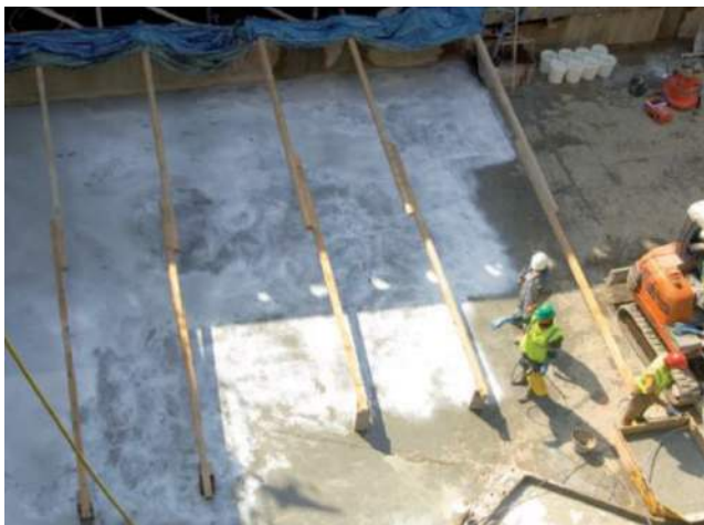
Fig. 6.11c—Placing UHPC in Caderousse Dam Spillway by pump (photo courtesy of Lafarge).
